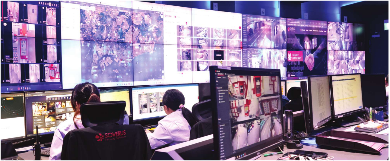
Secura Integrated Command Centre (SICC)
